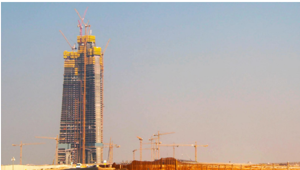
Fig. 20. The building site of the Kingdon Tower in Jeddah at the beginning of 2018.
