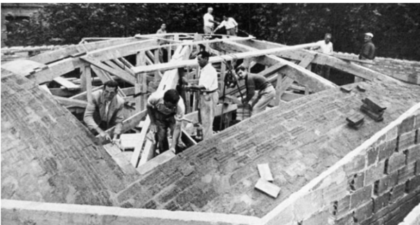
Fig. 1. Construction of Catalan vaults for the Sagrera Market in Barcelona [Torroja 1957, p. 280].
