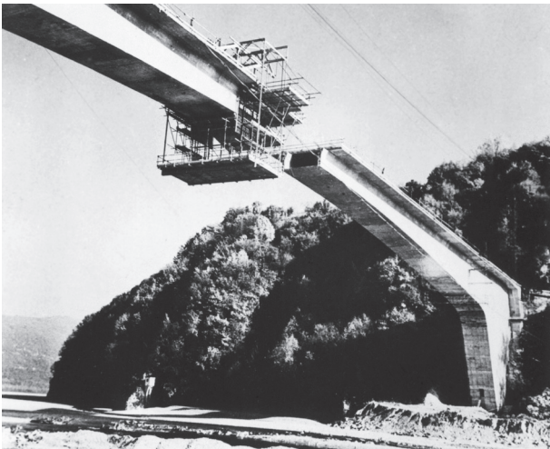
Fig. 10. Bridge over the river Tagliamento at Pinzano, under construction (Historical Archive of the Politecnico di Milano, Silvano Zorzi Collection, Milan).
