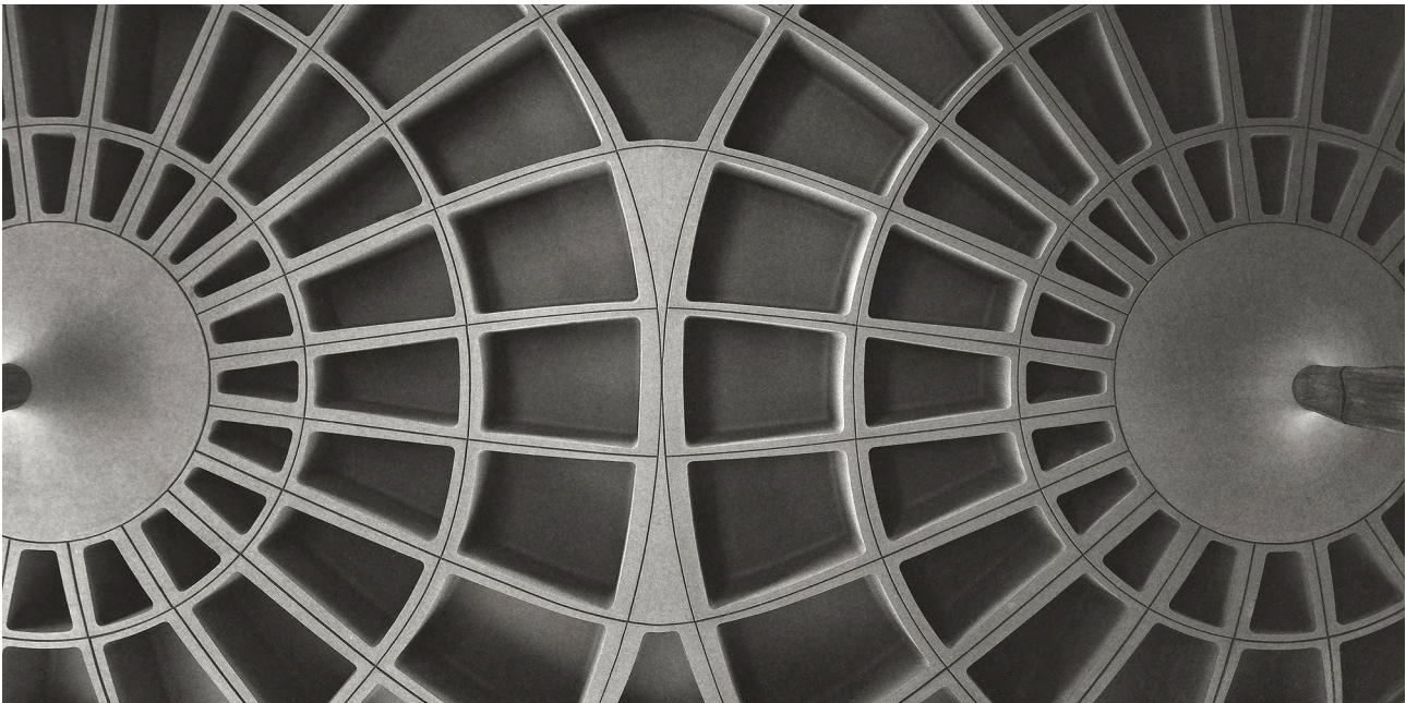
Fig. 14 Photograph of the underside of the roof of the church Cuore Immacolato di Maria in Borgo Panigale (photo @ Matteo Cirenei).
