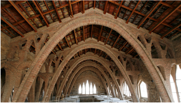
Fig. 1. Detail of the main beam of the Pinell de Brai Cooperative, built with brick arches. Image credit: Department of Culture of the Generalitat de Catalunya.
