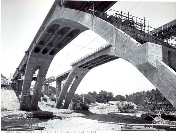
Fig. 7. Bridge on the Autostrada del Sole at Incisa, under construction (In.Co. S.p.A. Historical Archive, Milan).
