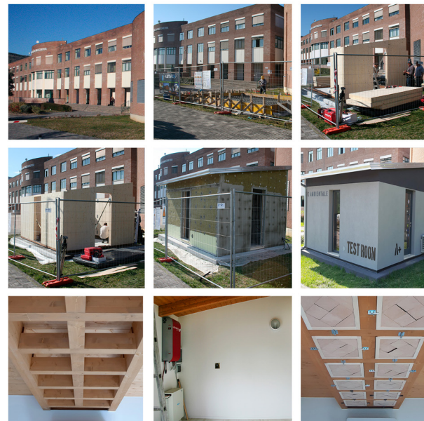
Fig. 8. Execution and installation of the test room for simulated performance verification graphic (graphic elaboration by the authors).
